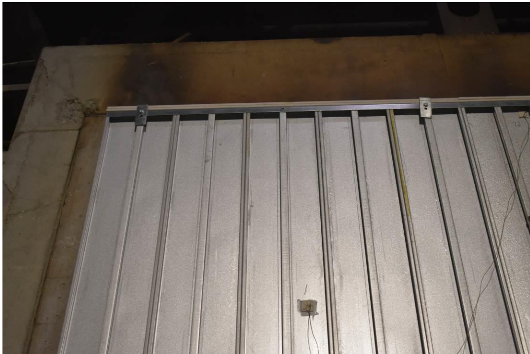
Photo No. 14 Discoloration of joint no. 4 seen from fixed edge
