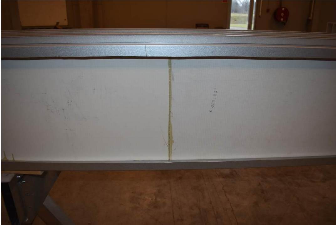
Photo No. 3 The glued joint in a M4 composite board during set-up at the sponsors location
