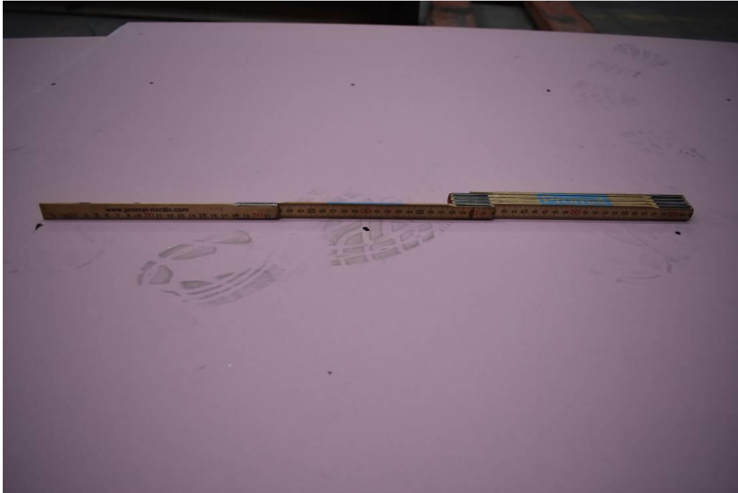
Photo No. 9 The gypsum plaster boards were mounted with screws cc 300 mm at mid width
