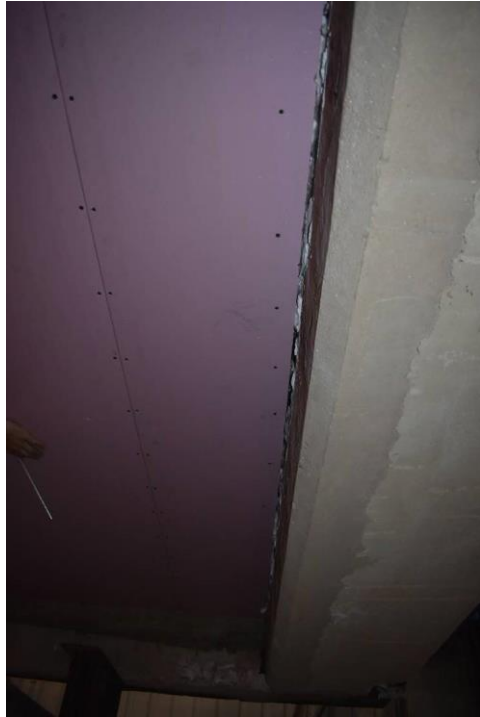
Photo No. 11 The first layer of gypsum plaster boards with width 400 mm by one end
