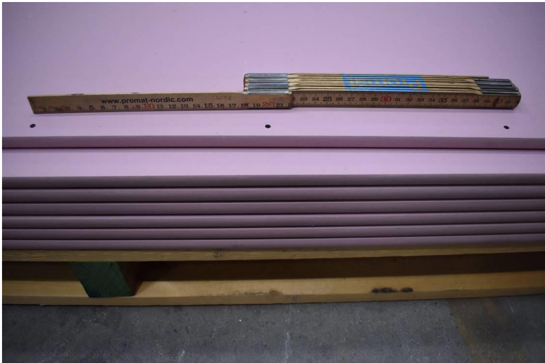
Photo No. 8 The gypsum plaster boards were mounted with screws cc 200 mm along the edges
